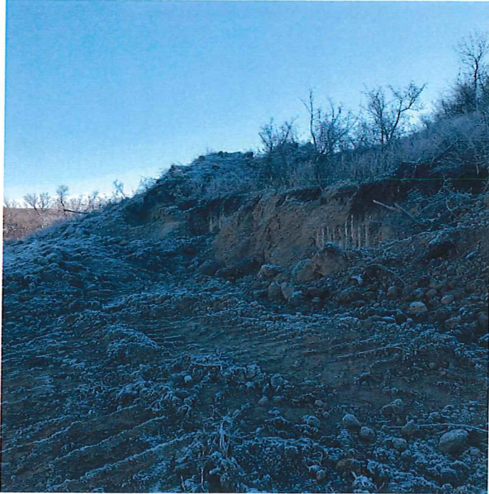
P35 – STA 55+15 BK_Grading Required
