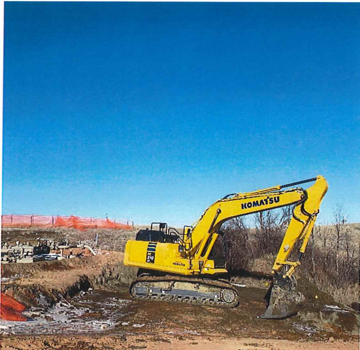
P44 – Equipment Onsite
