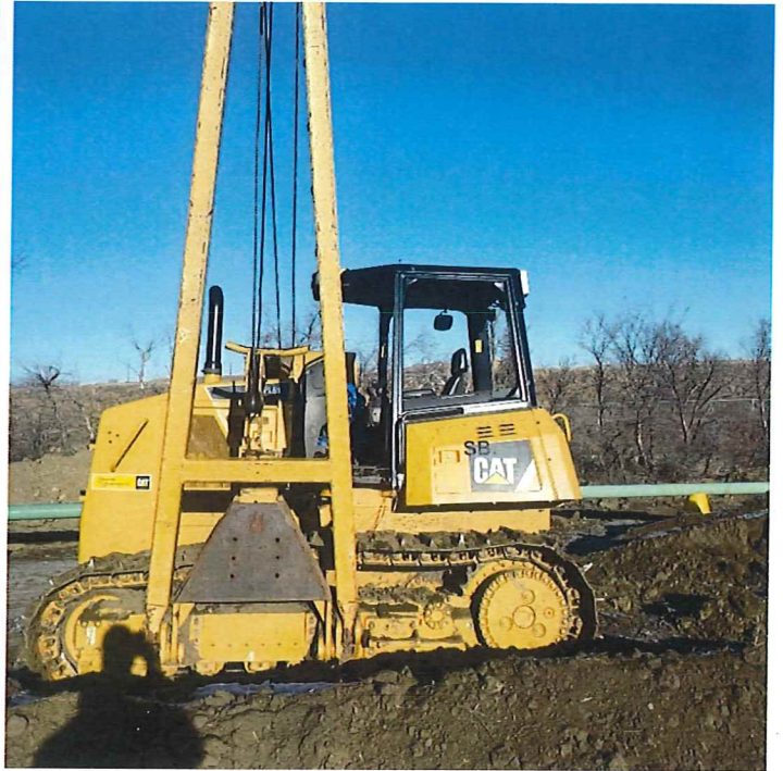
P43 – Equipment Onsite
