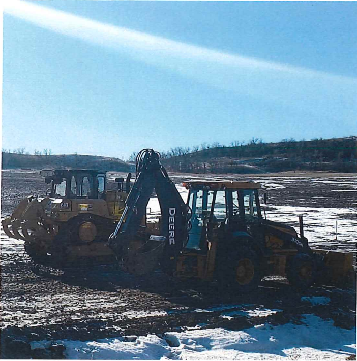
P42 – Equipment Onsite
