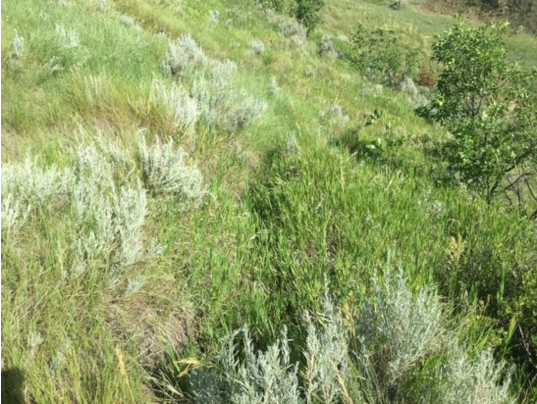
Photo Type: Slope movement evidence | Photo Bearing: 306 degrees Photo Description: Looking at a possible tension crack near top of slope.
