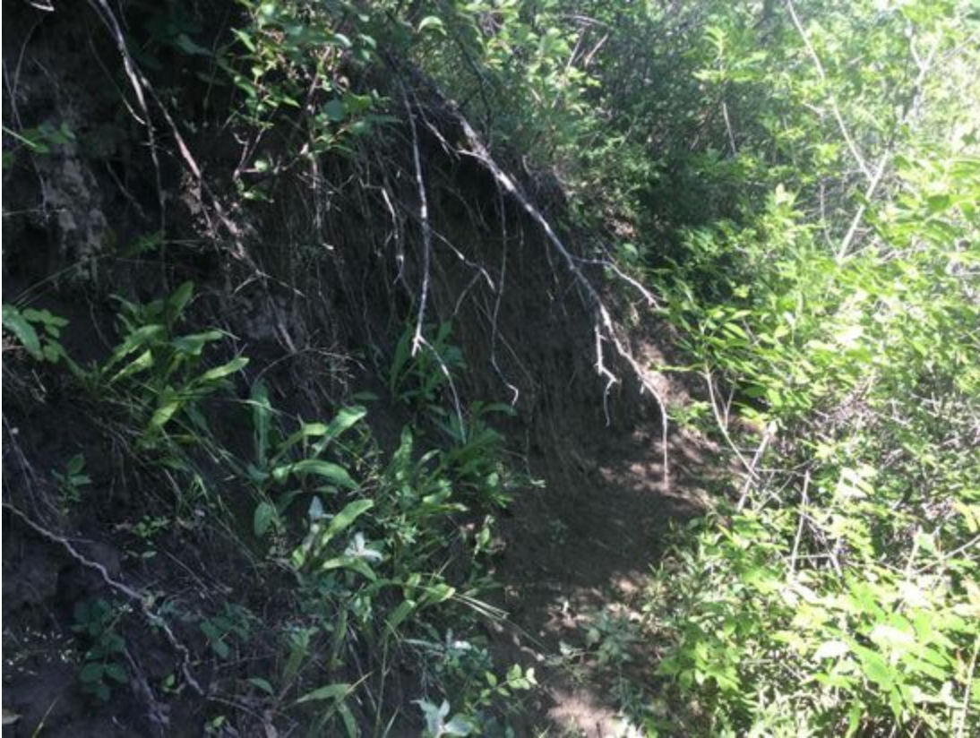
Photo Type: Slope documentation | Photo Bearing: 265 degrees Photo Description: Oversteepened section of the north-facing slope at historic slide head scarp.
