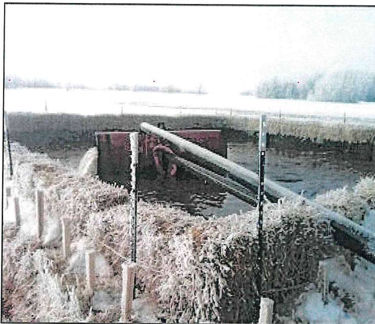
Hydrostatic Test Water Discharge Structure
