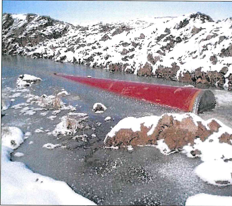
Trench With Frozen Infiltrated Groundwater
