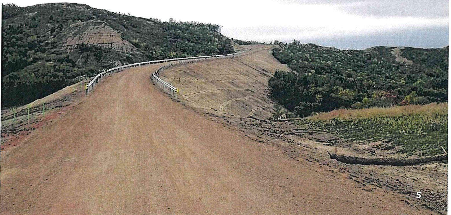
Example of construction and reclamation of an access road during and after construction.
