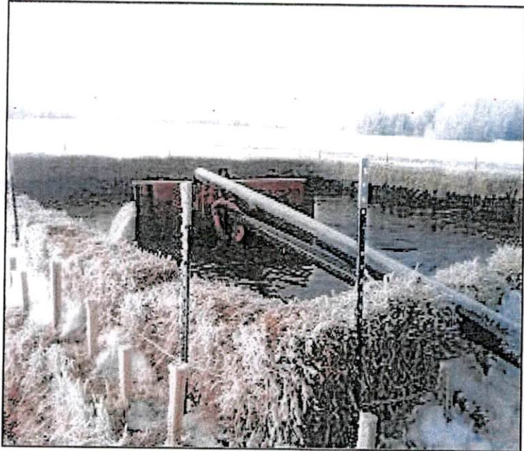
Hydrostatic Test Water Discharge Structure
