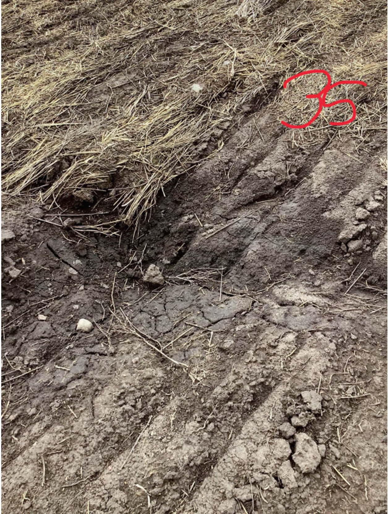
P35 looking SE, localized sink in farm field, however, landowner was working land anyway.
