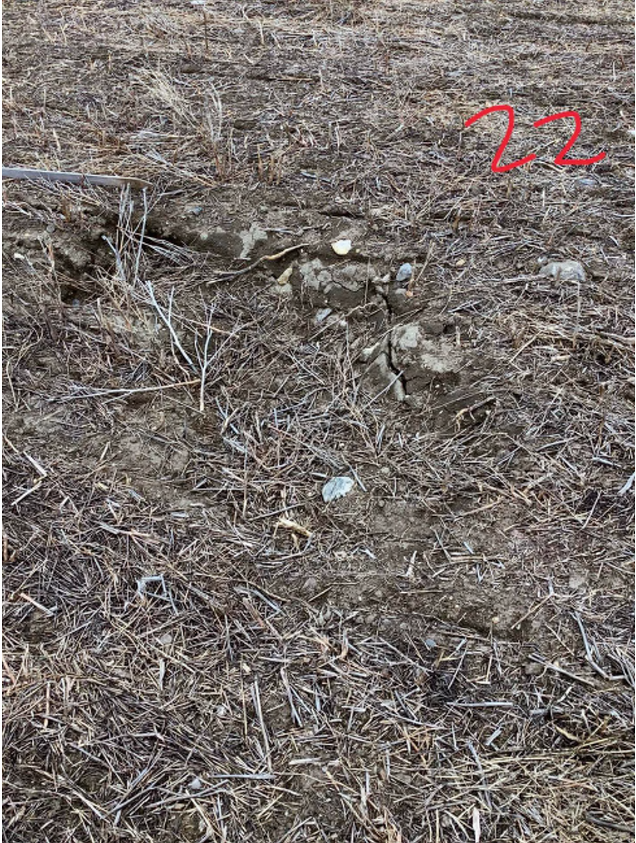
P22 looking SW, localized trench sinkage and soil cracking.
