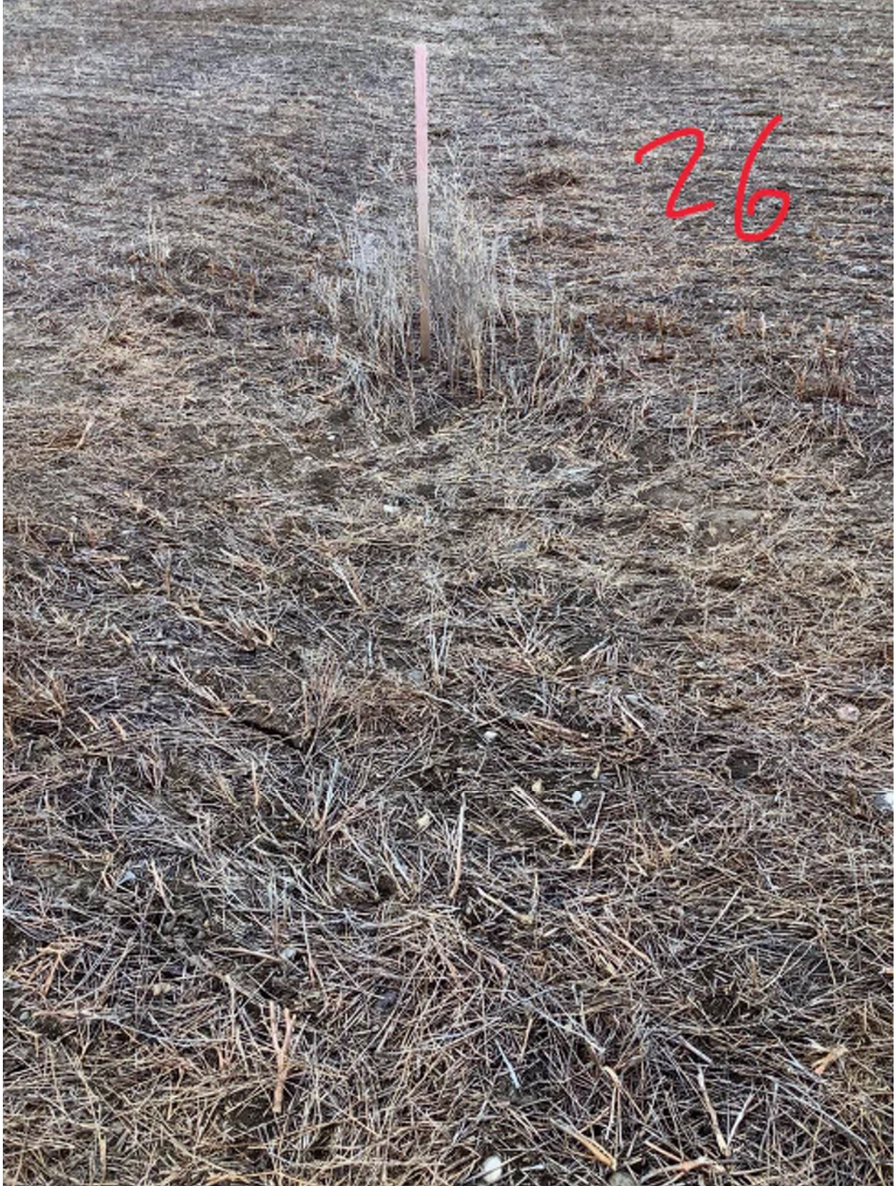
P26 looking SW, minor trench sinking along ROW. Landowner has been utilizing the area.
