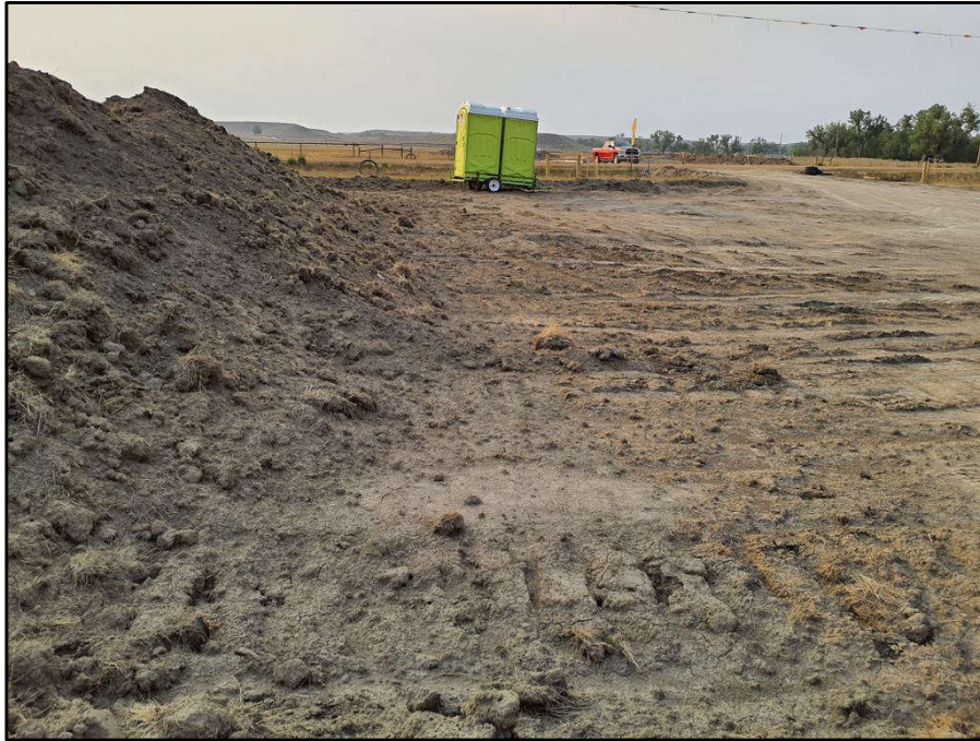
Figure 11. Overview of the current pipeline blading activities adjacent to addition 3, facing northwest.
