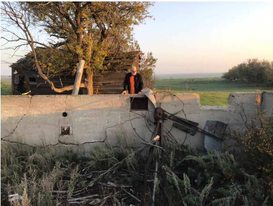
Figure 36. Site 32LO165 Feature 1 overview of farmstead foundation with coal chute and exhaust ducting.
