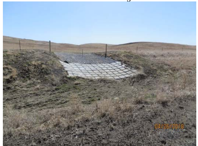
NAC lowered the berm by the fence. This lowered berm provides a path for water to flow from NAC land onto the Farmland which created gullies.
