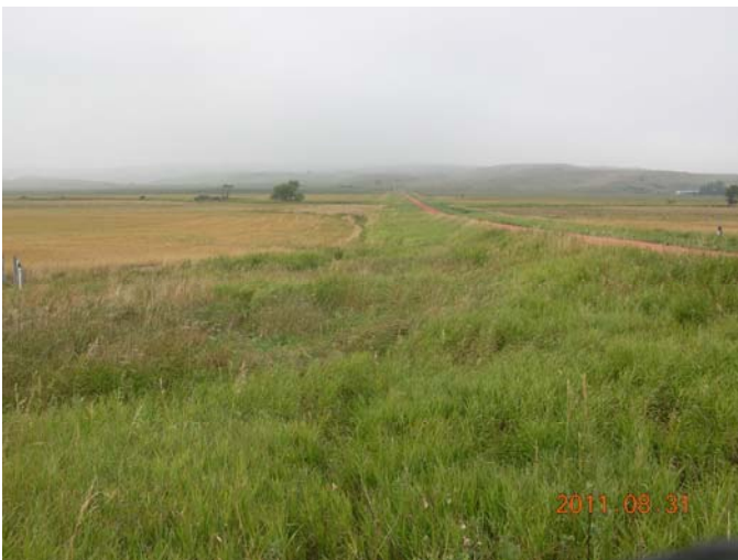
Original road ditch with Pond water overflow erosion visible on far end.
