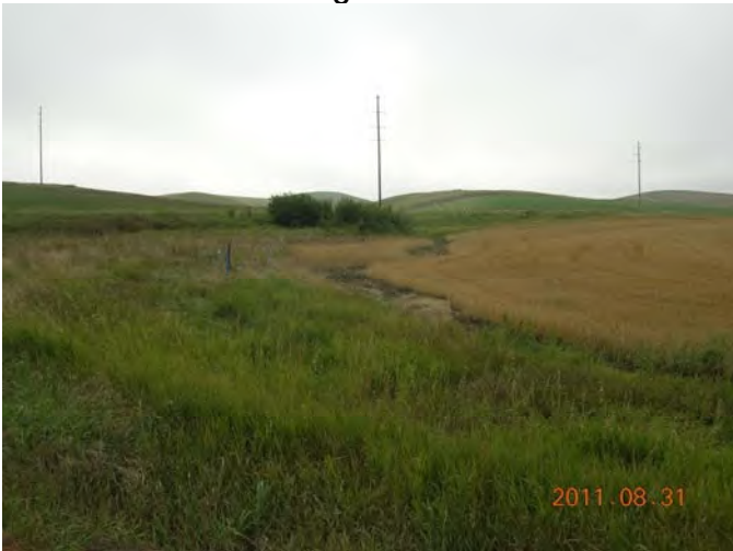
Pond water overflow erosion between original diversion ditch and original road ditch .
