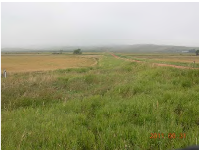
Original road ditch with Pond water overflow erosion visible on far end.
