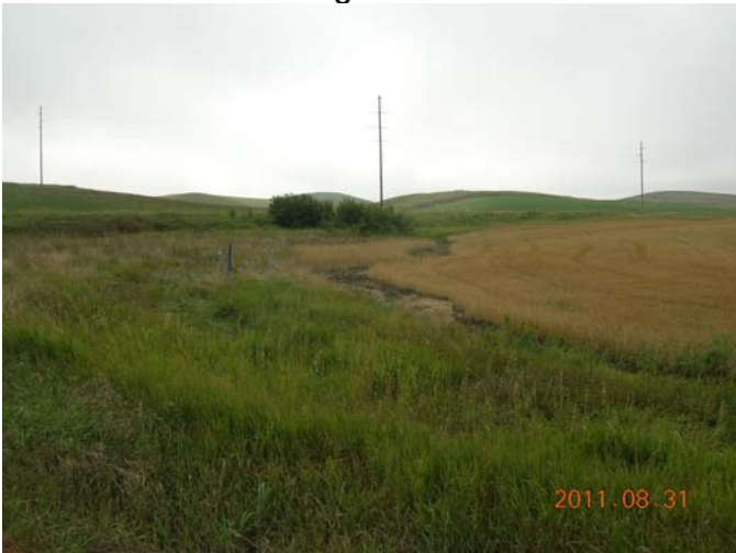
Pond water overflow erosion between original diversion ditch and original road ditch .
