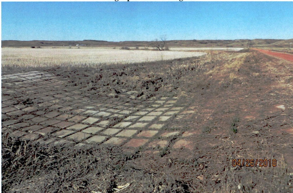
Figure 3. Flexcrete crossing in the road ditch on the north side of the NW¼ of Section 34. Photograph taken facing west.
