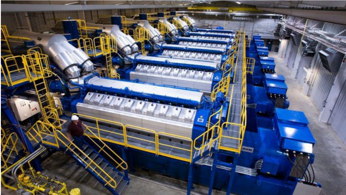
Figure 2-9: Engine Hall at Goodman Energy Center in Kansas
