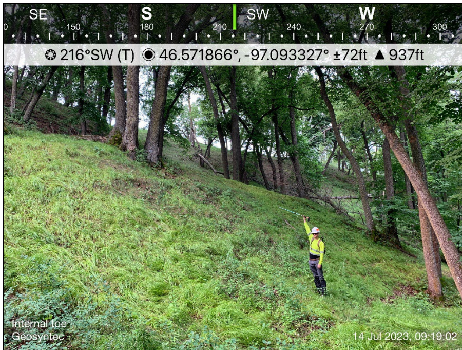
View facing southwest at an internal landslide toe that was approximately 10 feet high and located approximately 150 feet west of the proposed pipeline centerline.
