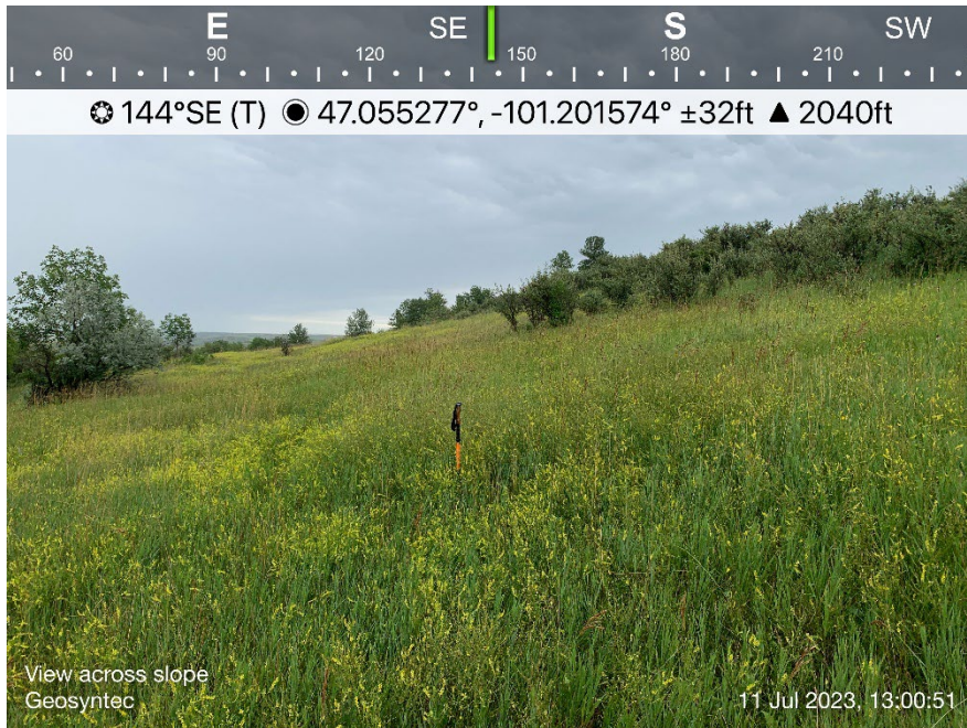
Looking southeastward across the body of the landslide mapped at Site #2. The proposed pipeline centerline is located out of view at the top of the slope to the right of the photo.
