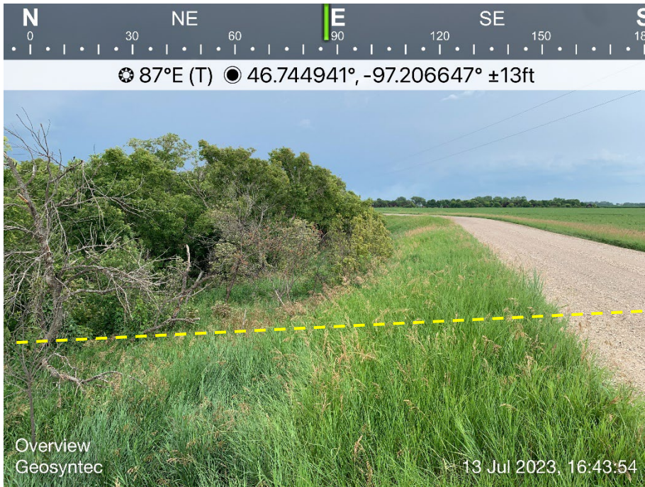
Looking east along the slope in the vicinity Site #14. The approximate proposed pipeline centerline is located near the center of the image (dashed yellow line). The proposed pipeline centerline crosses a possible recently active bank slump in the left portion of the image. Note the road was undisturbed.
