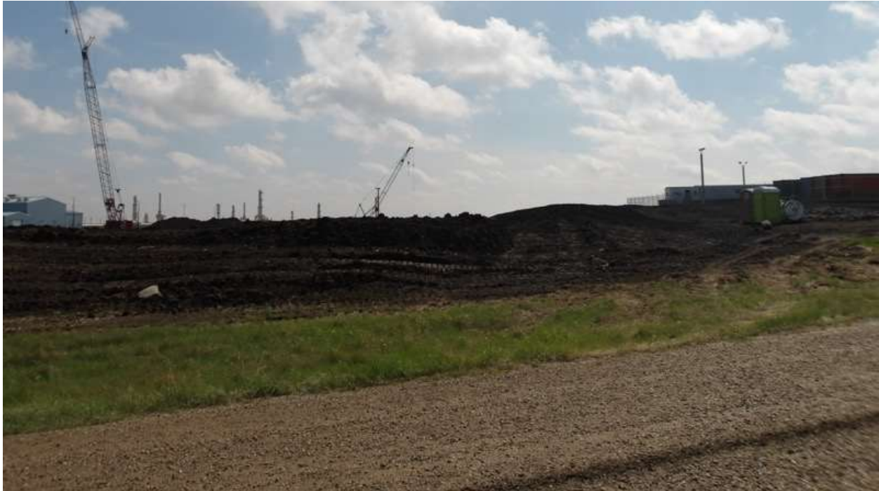
Figure 4: Construction area along the Pioneer to Judson 345 kV transmission line project area, view north (Image #SMT_215, 5/27/23)
