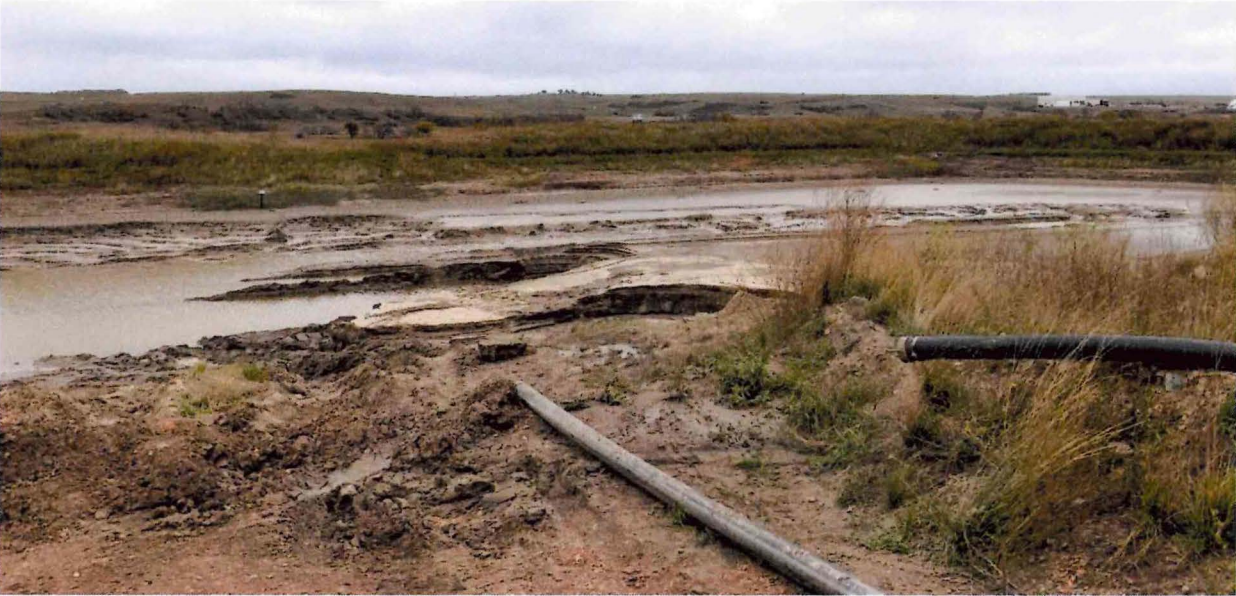
Figure 1: Sedimentation Pond P30-02 located in the NW¼ of Section 30 was observed to have sediment within the pond basin. Pond P30-02 was previously dredged in the summer of 2023 but the dredger was unable to successfully remove all of the sediment; therefore, CCMC plans to utilize a long reach backhoe to remove the remaining sediment.
