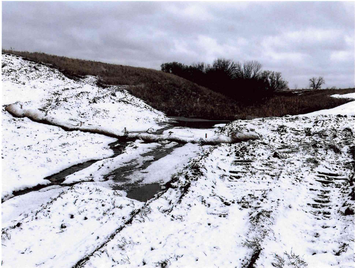
Figure 1 – Upstream end of reconstructed drainageway within grade approved area Gold-01-2022 — (looking southwest) in Permit KRSB-8603.
