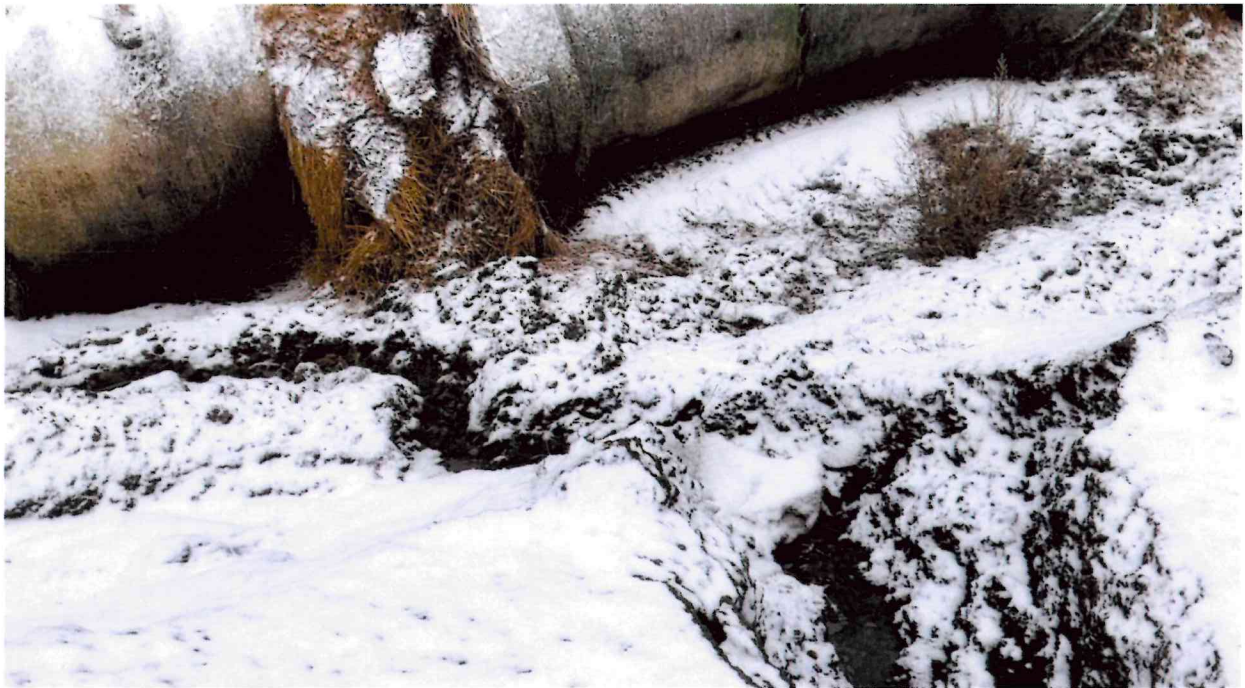
Figure 5 – Erosional feature immediately below the head cut and plunge pool.
