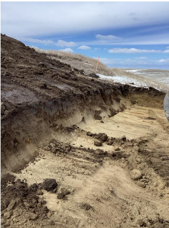
Point 8, Structure #366-058. Start of subsoil cut and clear line of soil type transition
