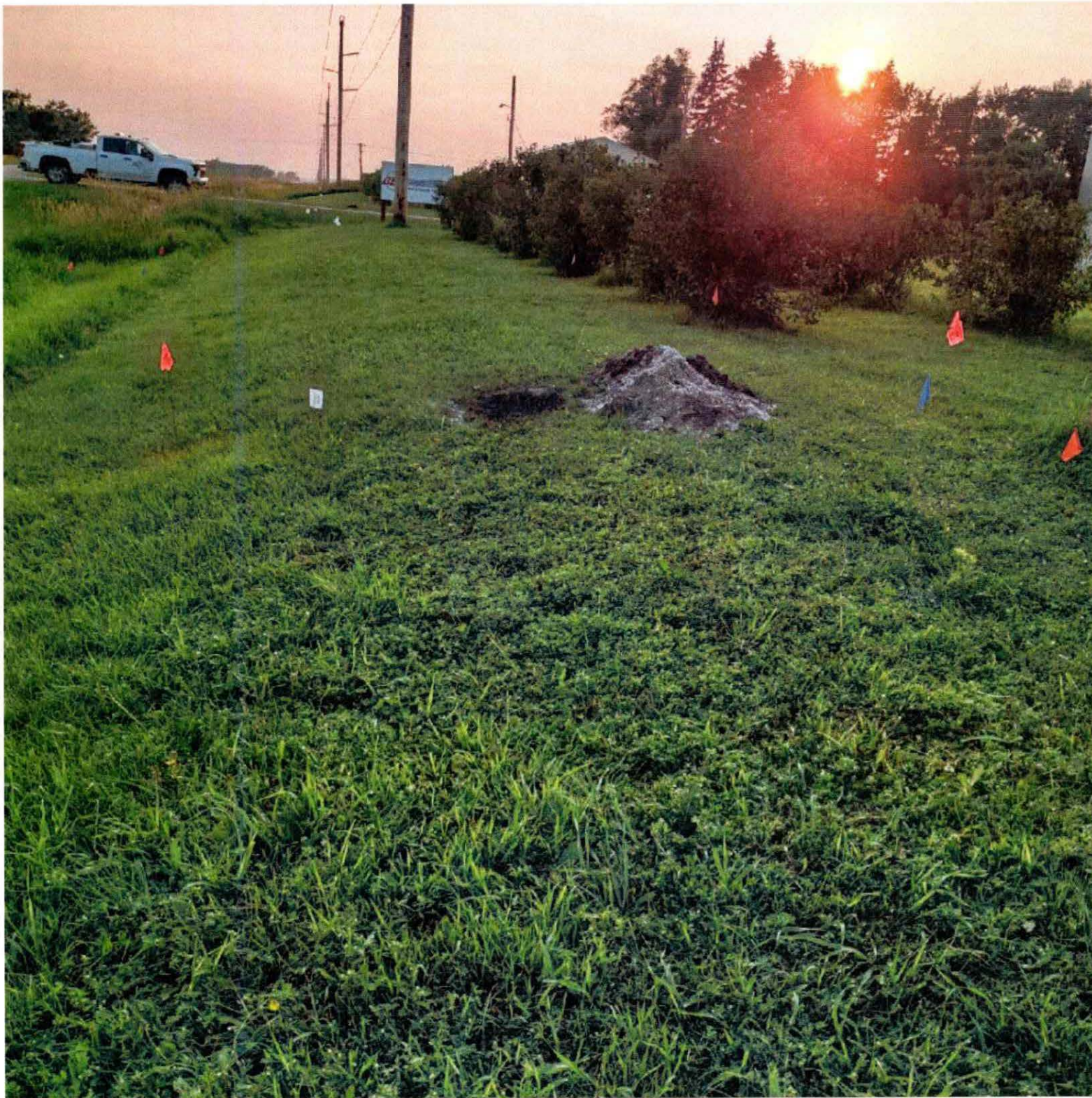
Pothole From finding other utilities
