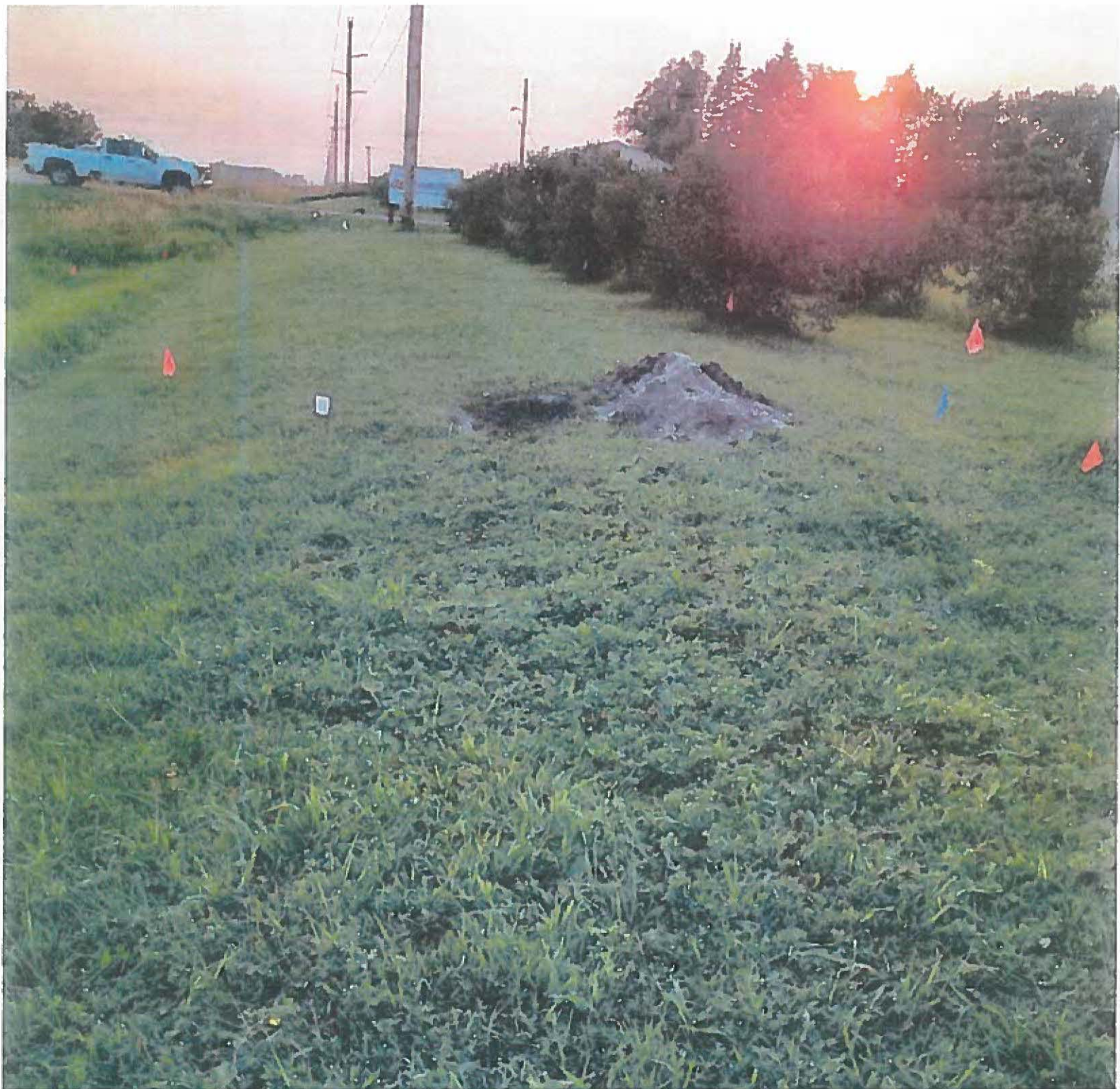
Pothole From finding other utilities
