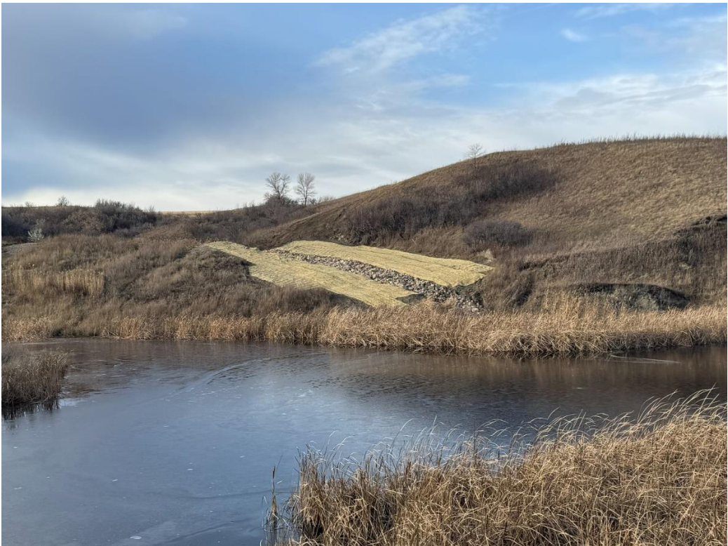
Figure 12: A rock channel was installed to replace a culvert with unstable, eroding soil.
