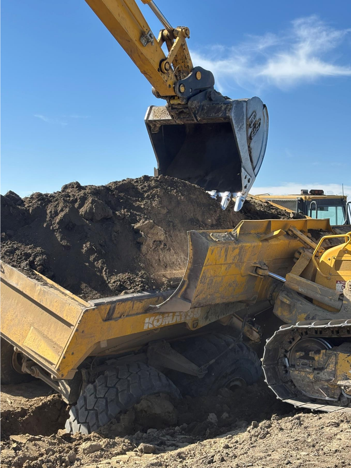
Figure 4: Over 17 inches of rain fell during the construction of the project, creating extremely muddy conditions.
