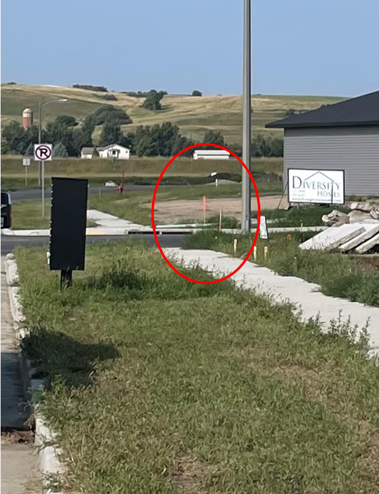
Photo 3: Stop sign not yet installed. The red circle shows lath stake painted pink is marking location of where the stop sign is to be installed.
