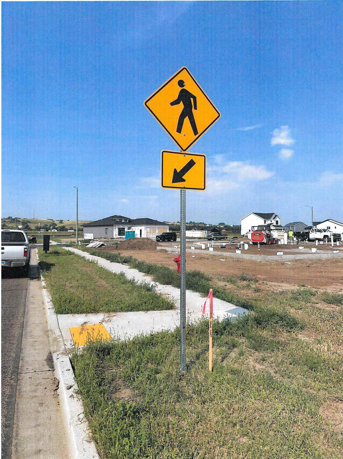
Photo 2: Closeup of North cross walk sign installed without on-call ticket.
