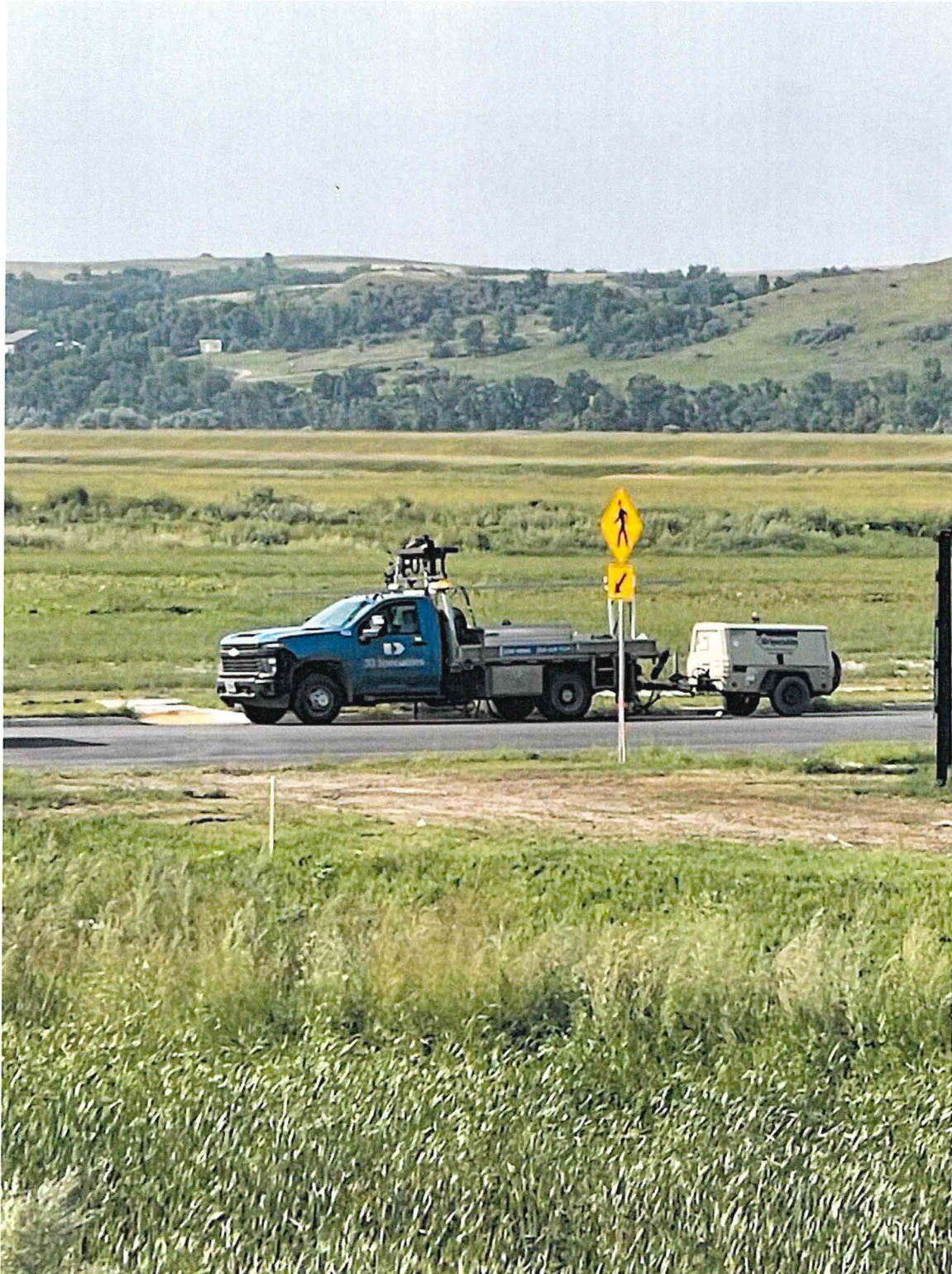
Photo 1: Dakota Fence at the location of installation with North crosswalk sign already installed.
