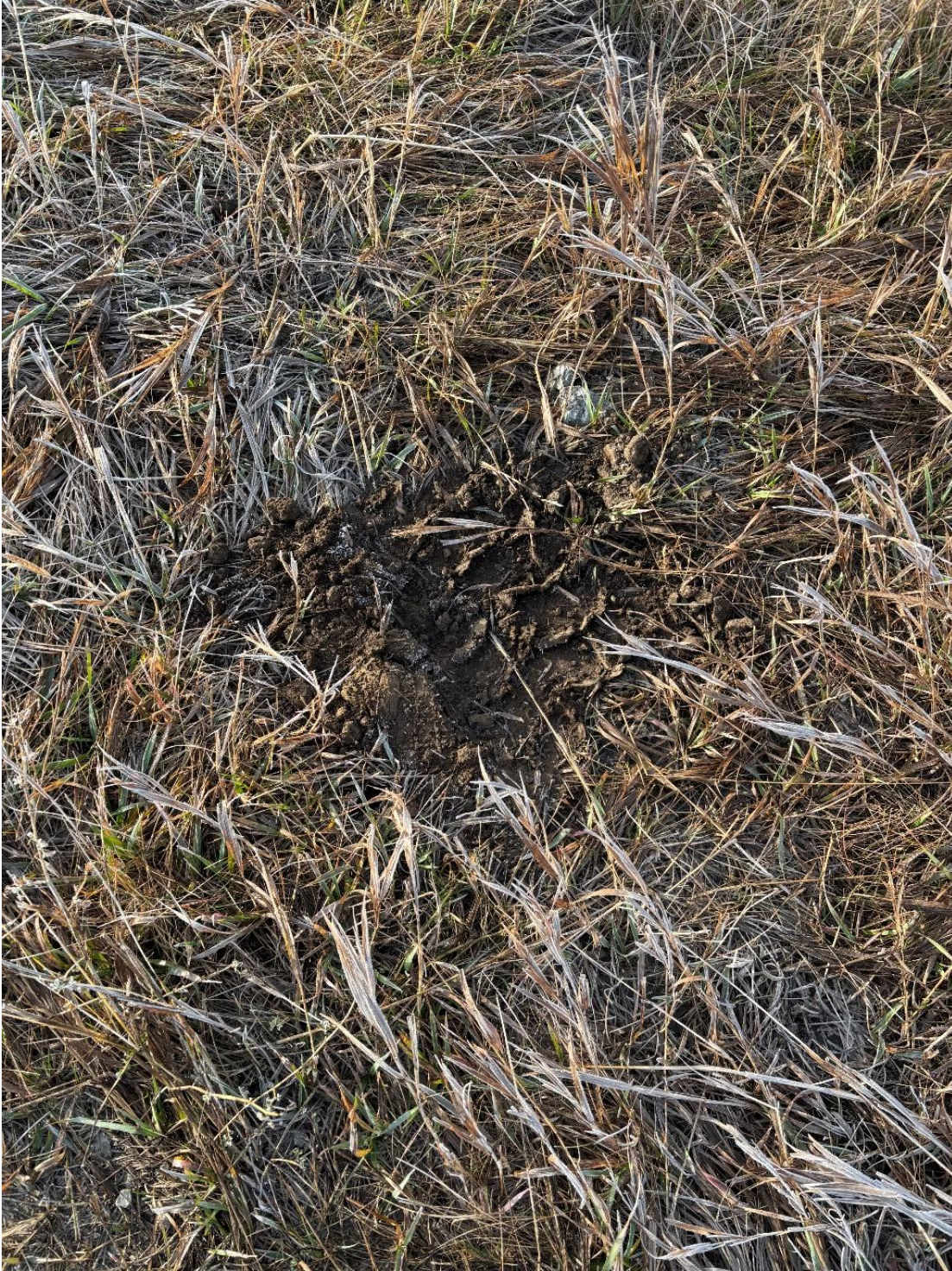
Figure 4 - WP18 – Improperly Finished Borehole
