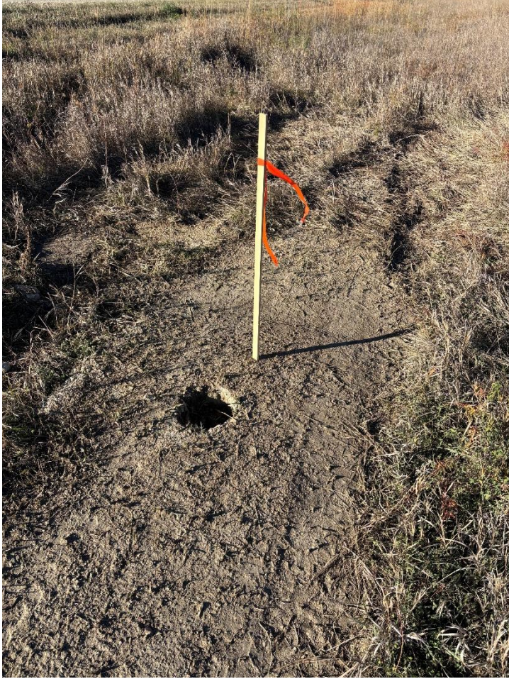
Figures 8 & 9 – An additional improperly backfilled borehole was found in the PSC’s follow-up inspection.
