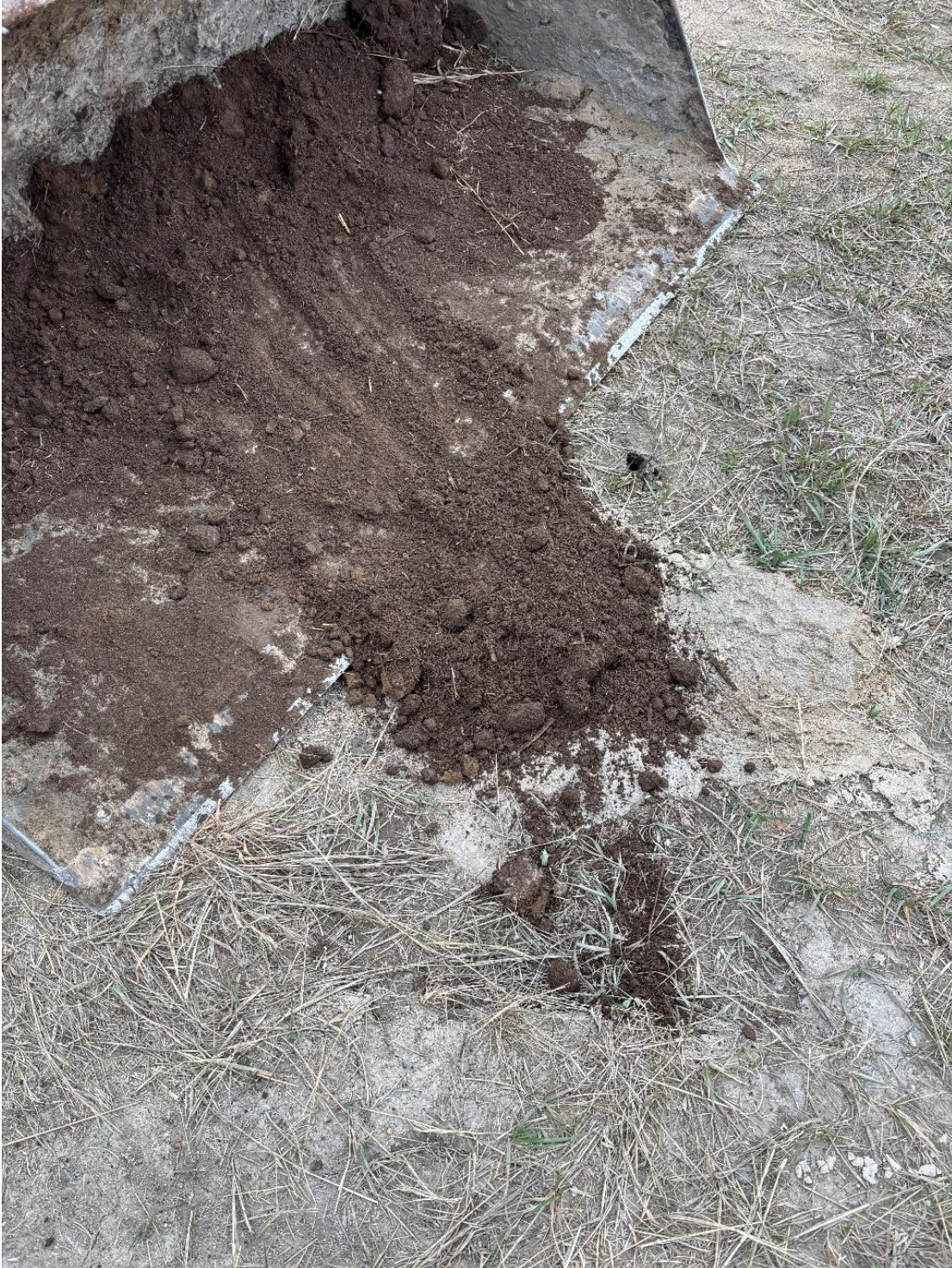
Figure 2 - WP16 – Improperly Finished Borehole
