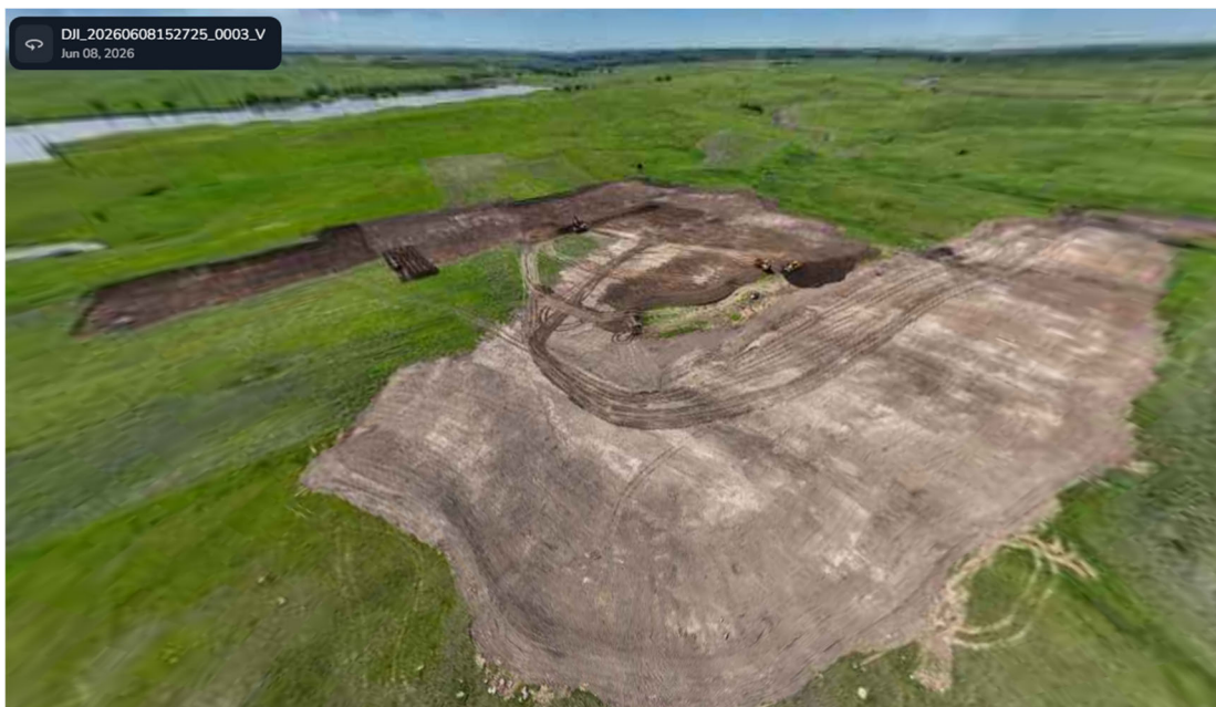
Photo 2: Nelson Lake Substation:
