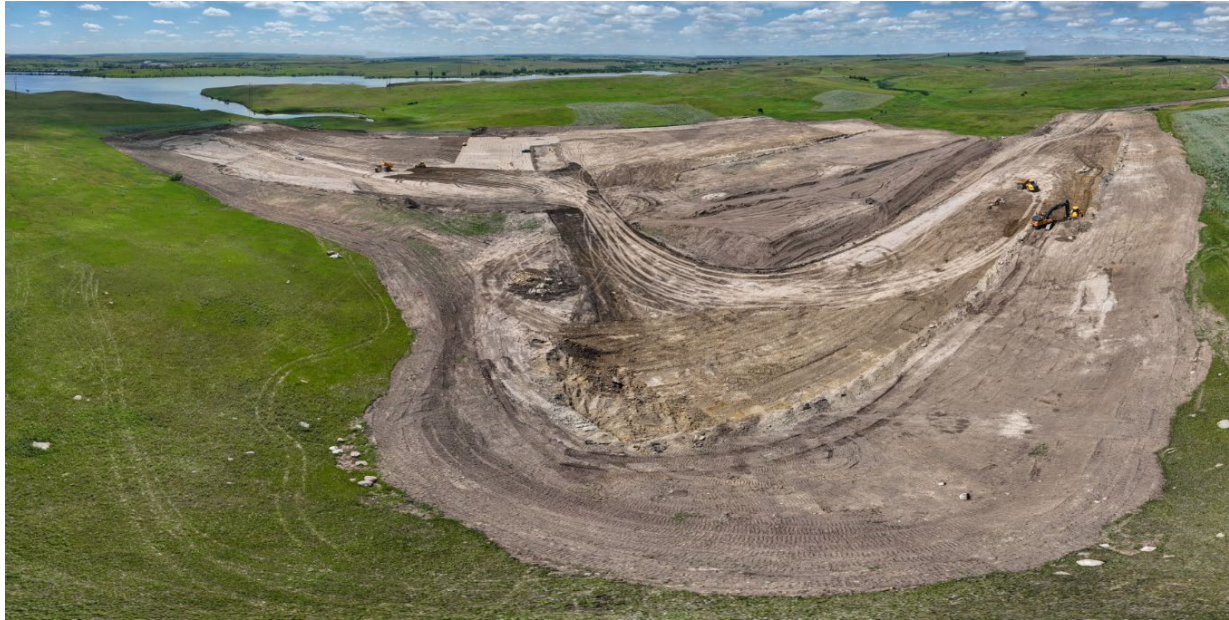
Photo 3: Nelson Lake Substation as of 7/8/26
