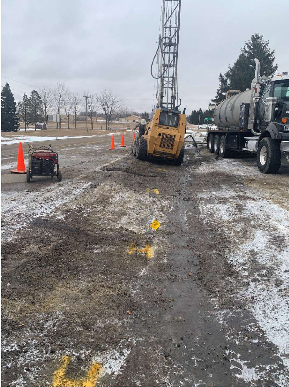
Figure 6 Yellow paint marks and pin flag showing the location of MDU's 4" plastic gas main.
