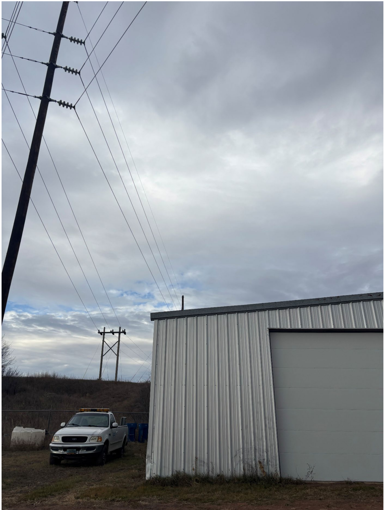
Figure 5: City of Beulah Storage Building (Power Line Insulation Location)
