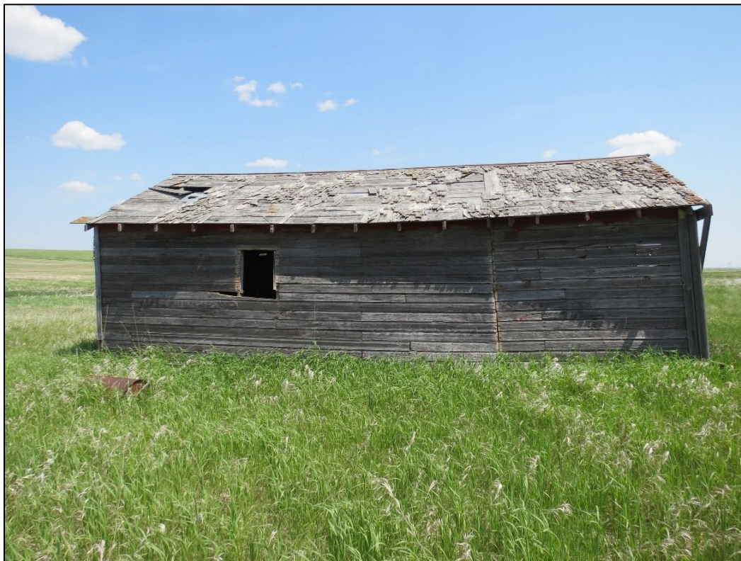
Figure 6-34. Feature 1- Side view of wood framed structure at 32WI2604. View looking east.
