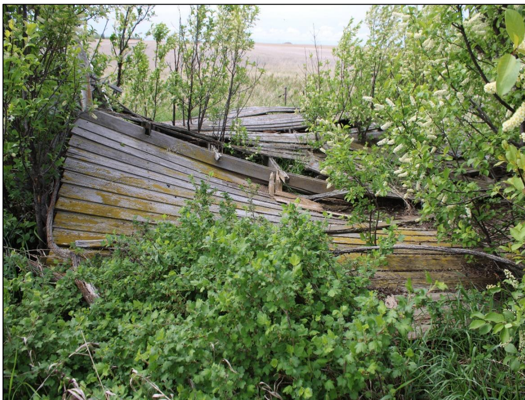
Figure 6-12. Feature 4- Collapsed wood framed structure at 32WI2593. View looking south.
