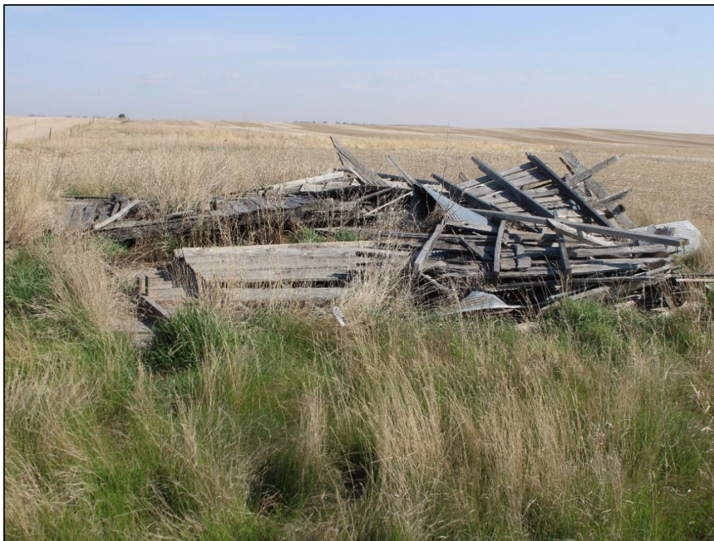
Figure 6-58. Feature 1- Collapsed wood framed granary at 32WI1704. View looking north.
