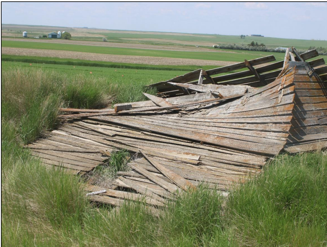
Figure 6-24. Feature 1- Collapsed wood framed structure at 32WI2596. View looking northeast.
