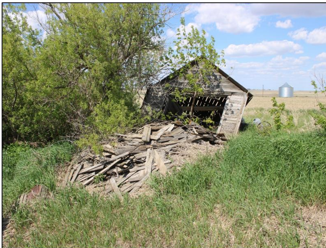
Figure 6-19. Feature 4- Partially collapsed wood framed shed at 32WI2594. View looking northeast.
