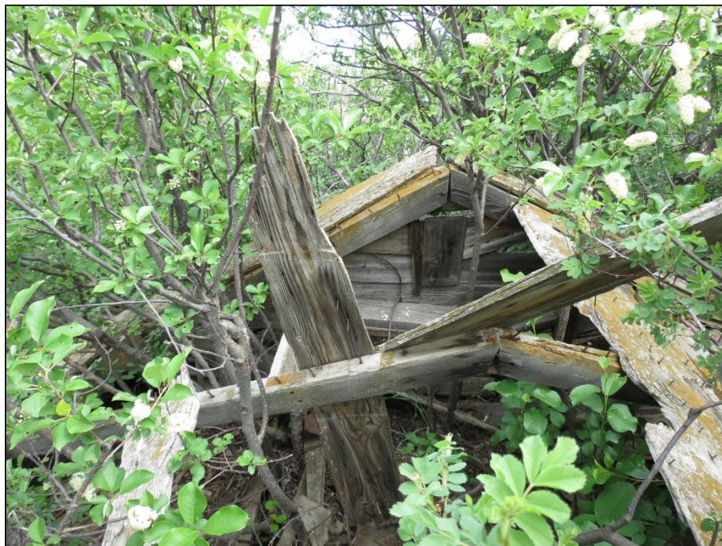
Figure 6-32. Gable apex of collapsed wood structure at 32WI2602. View looking northeast.
