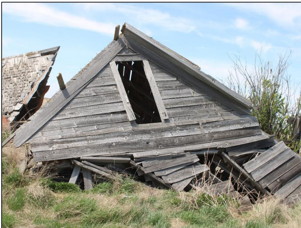
Figure 6-5. Feature 2- Collapsed wood framed house at 32WI2592. View looking west.
