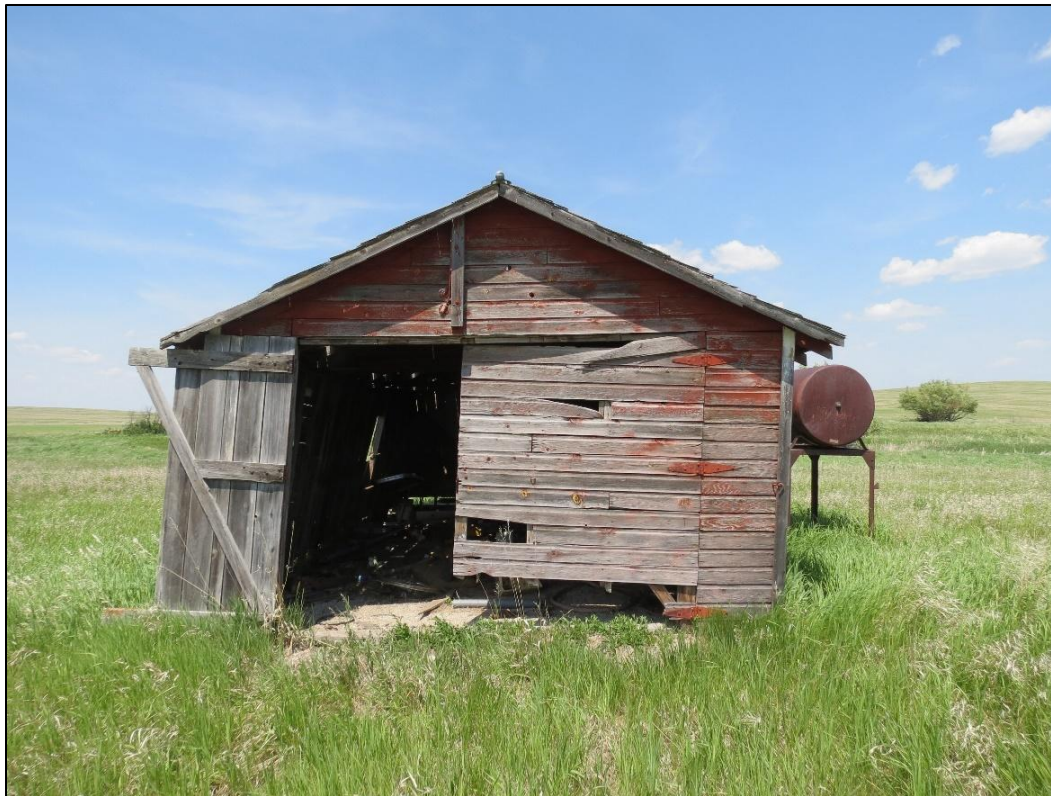
Figure 6-33. Feature 1- Frontal view of wood framed structure at 32WI2604. View looking north.
