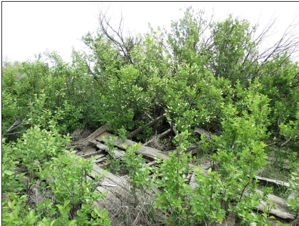
Figure 6-31. Collapsed wood structure at 32WI2602. View looking east.
