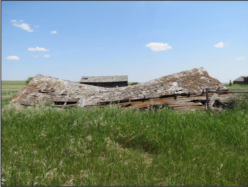
Figure 6-41. Feature 7- Side view of wood framed roof at 32WI2604. View looking east.
