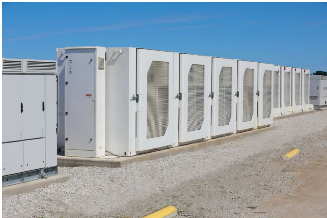
Image 3. Battery Energy Storage System Example
