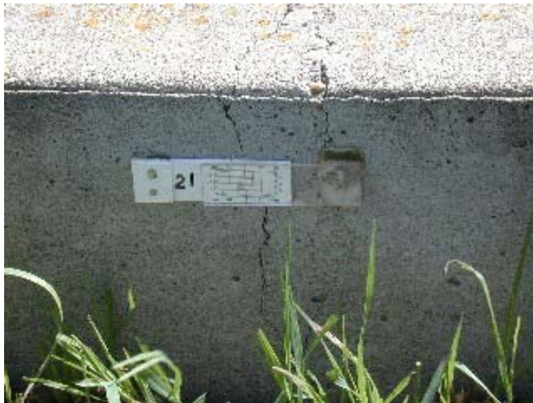
Figure 3: Crack Monitor installed on a crack in a retaining wall at the Beulah City Site.
