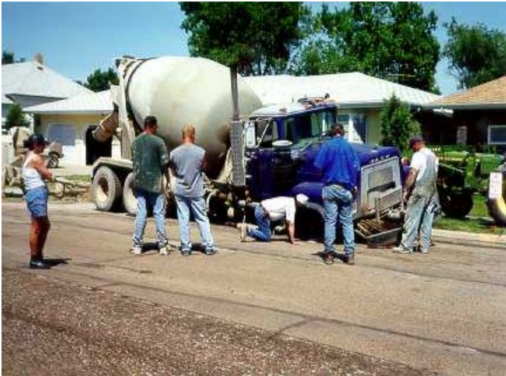
Figure 6: Loaded grout truck dropped its front wheel into a sinkhole on 1 st Avenue, Beulah
